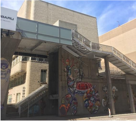
The (obscured) façade of the Commons on Champa Building. The elevator shaft and raised walkway will be removed in summer 2017.
